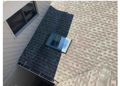
Unprotected glazed opening skylight
