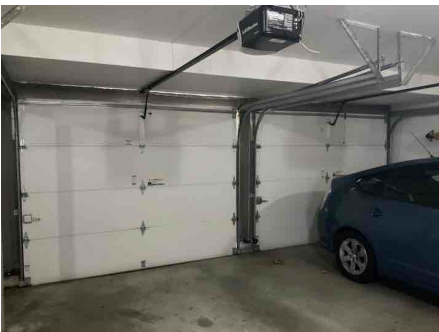
Unprotected garage doors
